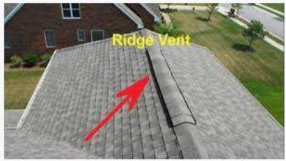
Ridge Vent System on My Roof ... emmonsroofing.com
